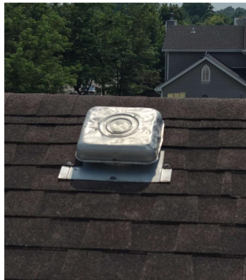
Damaged mushroom vent cap
