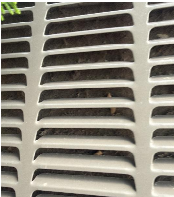
Vegetation Obstructing Condenser
