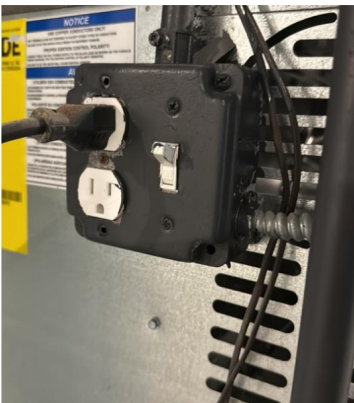
Service shutoff switch
