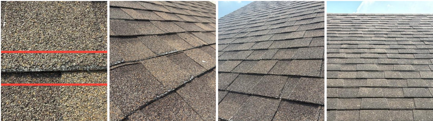
Significant granule loss around edges of shingles
