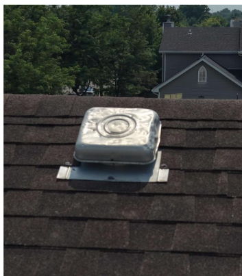
Damaged mushroom vent cap
