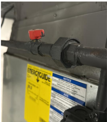
Furnace gas shutoff
